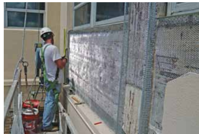
The scope of the 32 West Gore project increased significantly when Western discovered lath deterioration four inches deep—twice that originally anticipated. Swing-stage work requirements and ongoing tenant/guest access made safety a primary consideration. Both the finished project and Western process earned Orlando Health praise.
